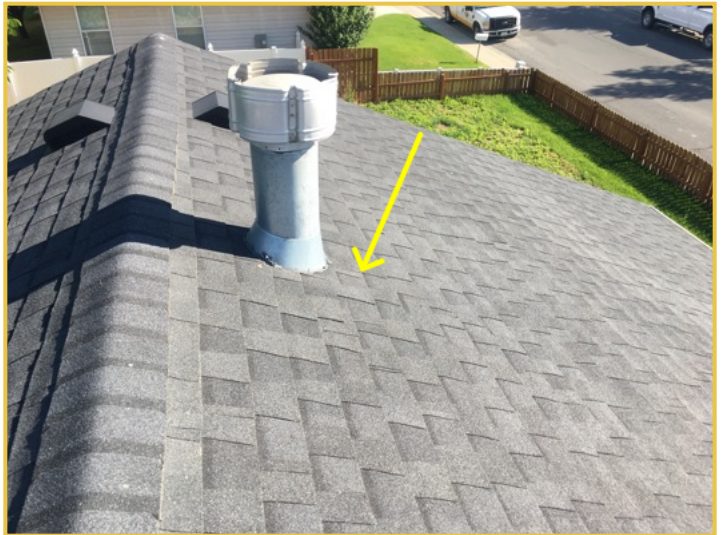
Improper Vent Flashing Installation
