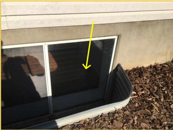
Condensation In the Basement East Window
