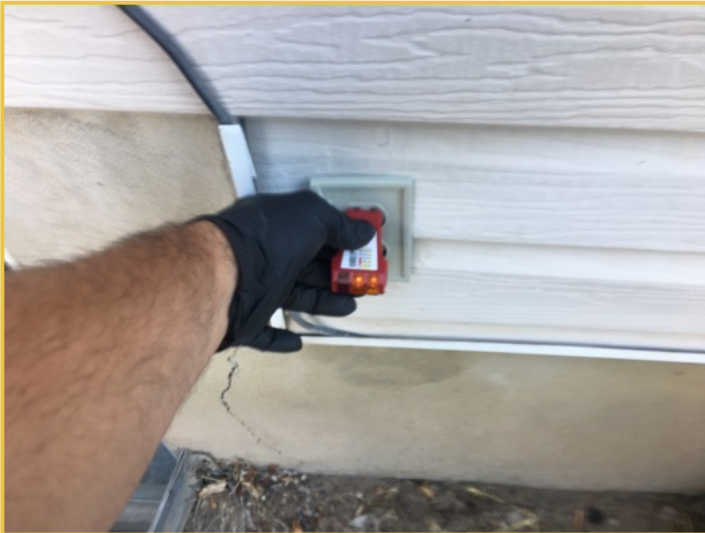
Exterior Outlets Not GFCI Protected
