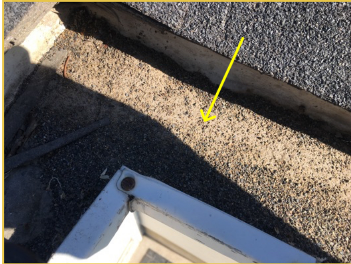
Debris in the Rain Gutters
