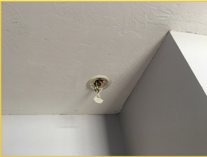
Missing Smoke Detectors
