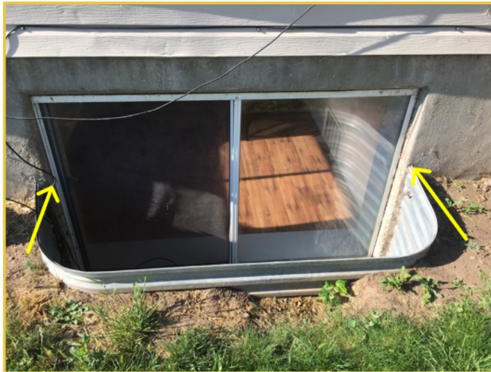
Basement Window Caulking Needed
