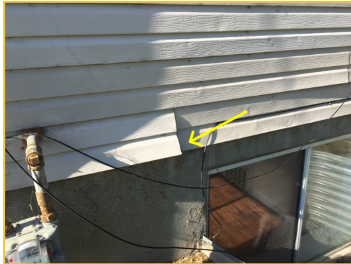
Damaged North Siding
