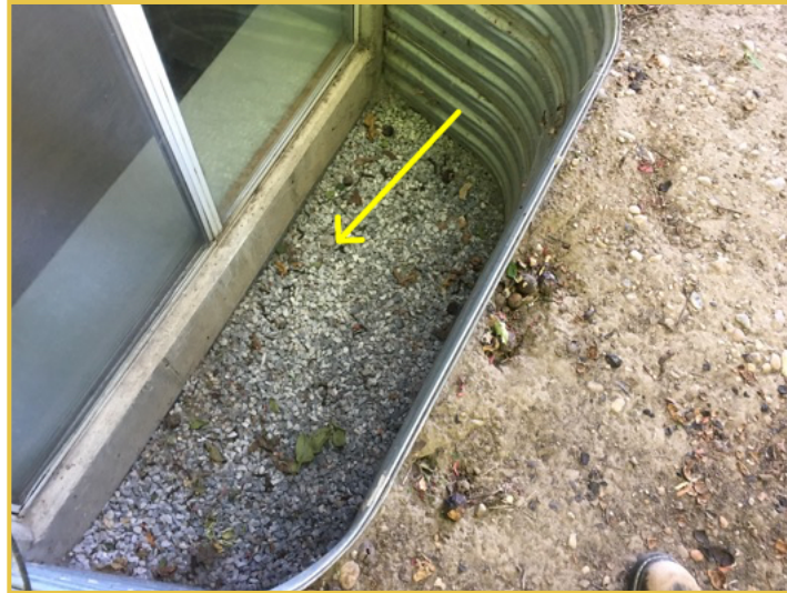
Window Well Grading Too Low
