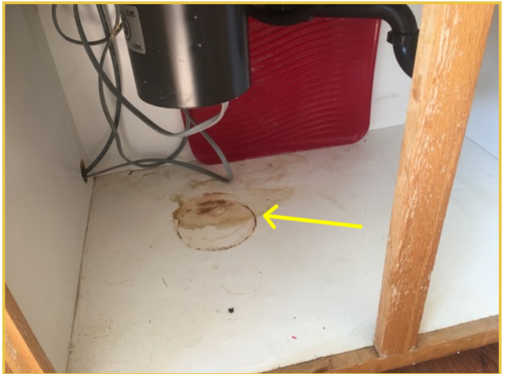
Evidence of Past Leaking at the Basement Kitchen Sink Under Cabinet
