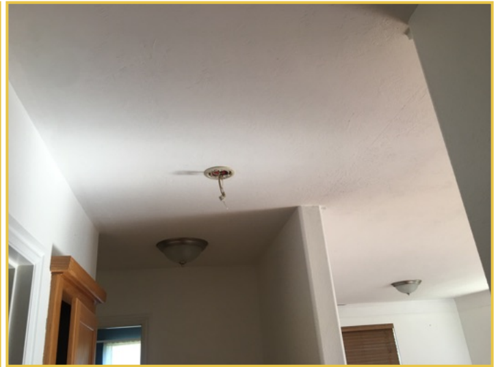
No Hallway Smoke/Carbon Monoxide Detector
