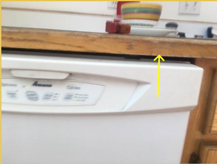
Main Floor Dishwasher Not Secured to the Counter Top or Cabinets
