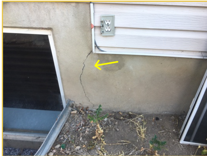
Large Foundation Crack
