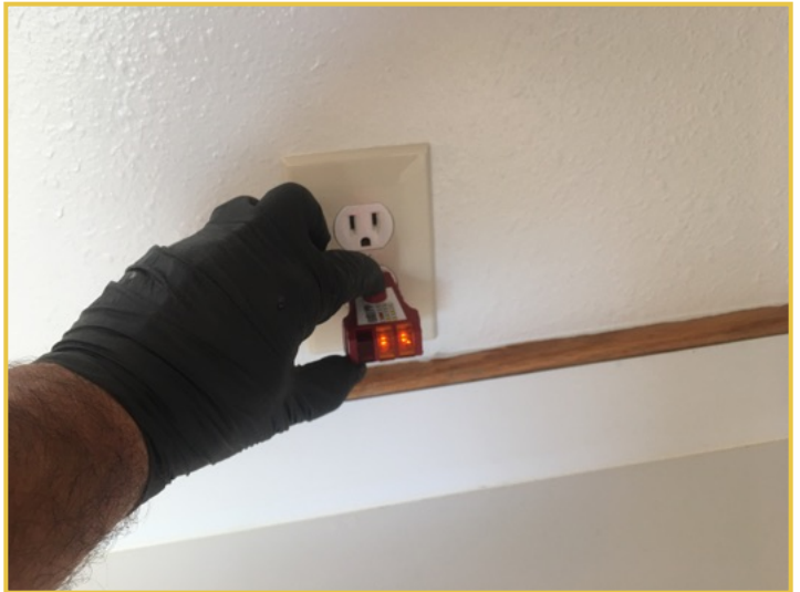
Basement Kitchen Outlets Not GFCI Protected
