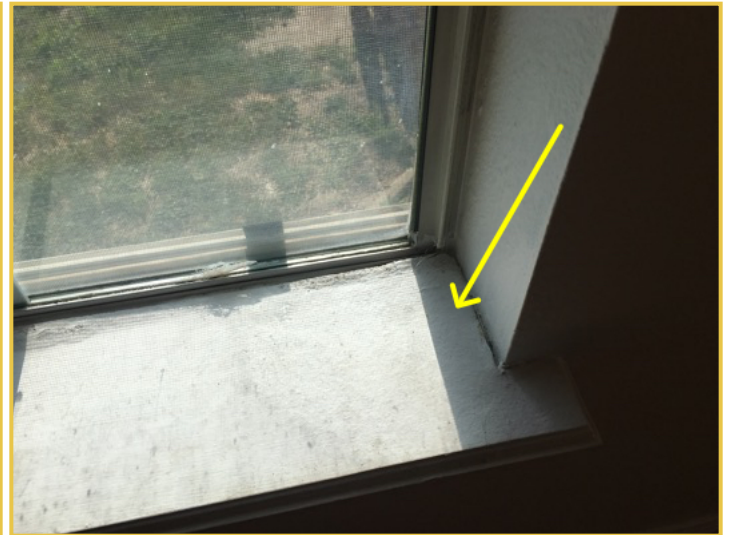
Evidence of Past Leaking at Several Window Sills That Was Dry
