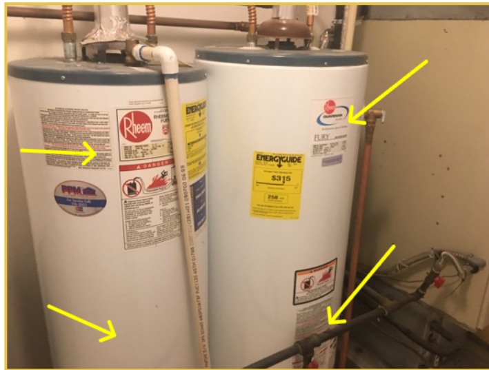
No Water Heater Earthquake Strapping
