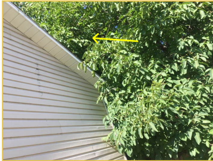
Tree Branches in Contact with the Roof
