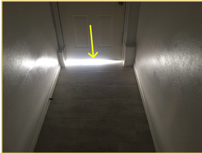
Missing Exterior Door Weatherstripping
