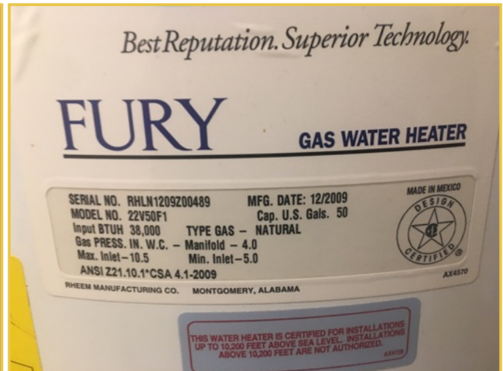
Water Heater Dated December 2009
