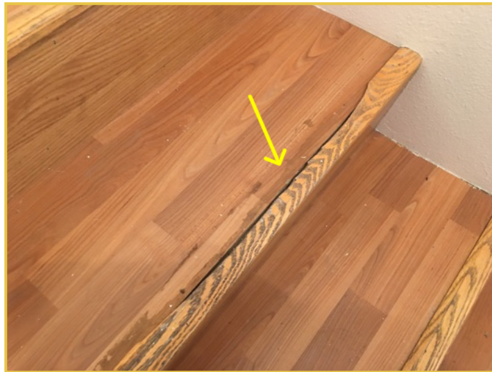
Damaged Stair Nosings
