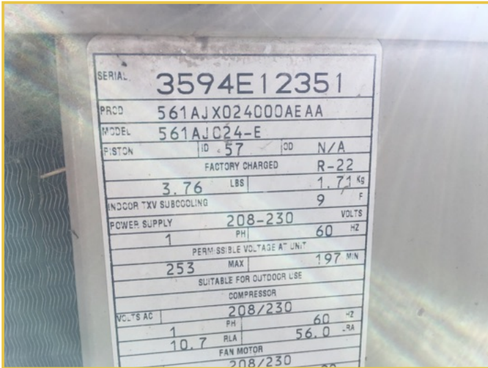
Main Floor Air Conditioning Condenser Dated September 1994
