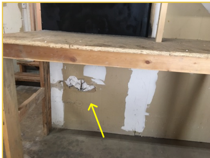
Holes in the Garage Wall
