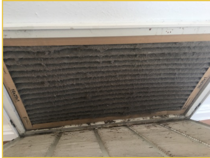
Dirty Air Handler Filter
