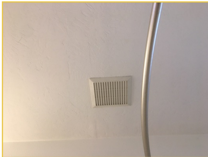
Main Floor Hall Bathroom Exhaust Fan Did Not Function
