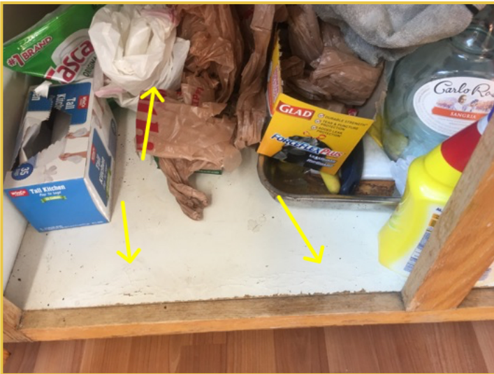
Evidence of Past Leaking at the Main Floor Kitchen Sink Under Cabinet
