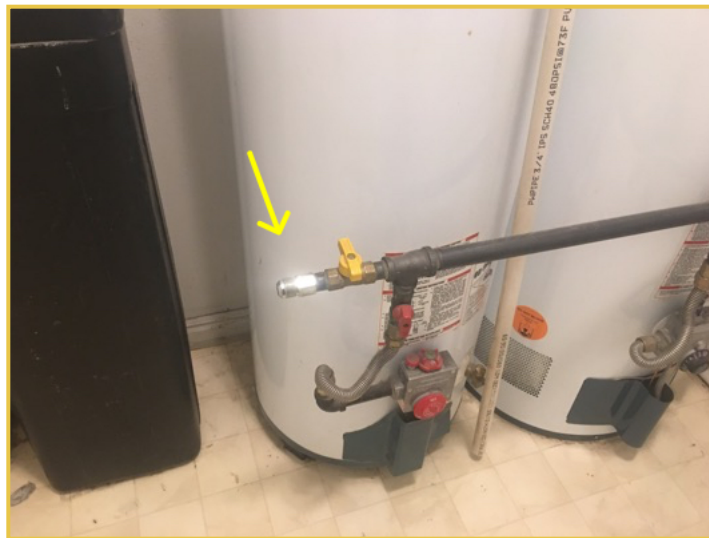
Utility Room Gas Line Should be Attached to an Appliance or Capped
