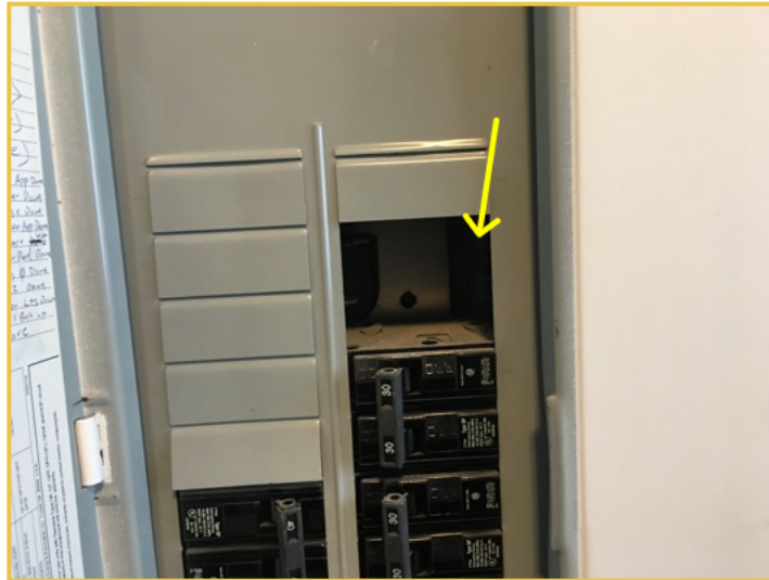
Missing Breaker Knockout
