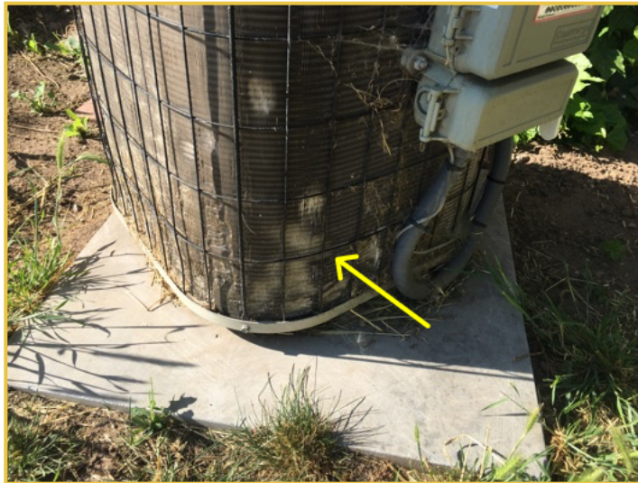
Air Conditioner Condensers Fin Damage
