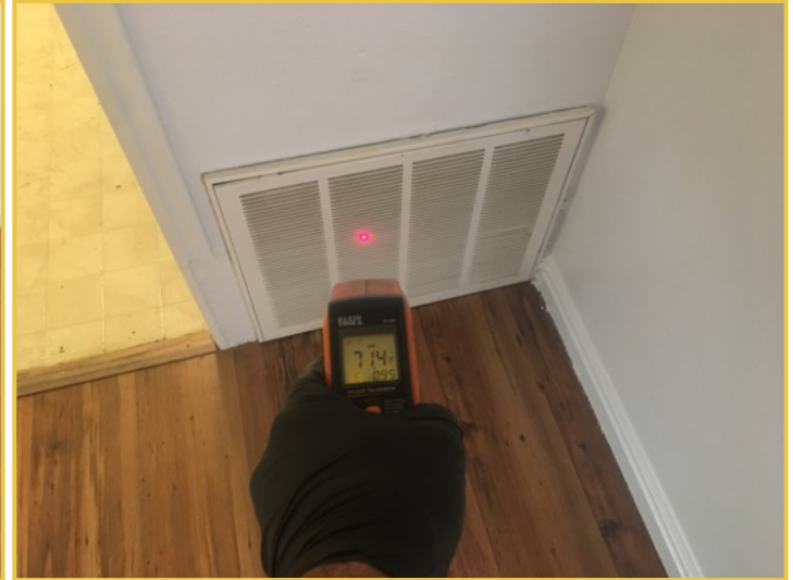
Basement Return Air Was at 71 Degrees
