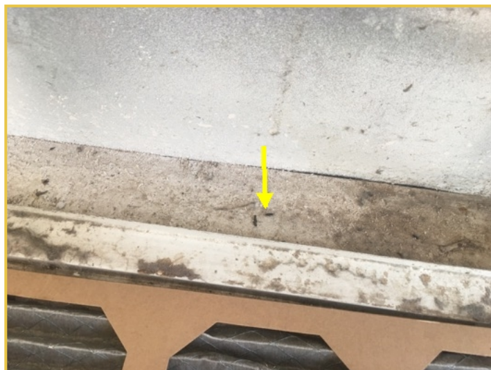
Rodent Droppings in the Basement HVAC Return
