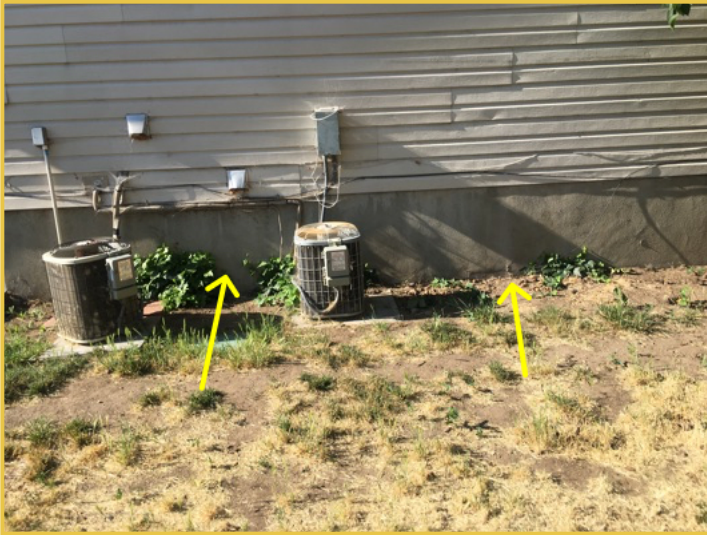
Improperly Sloped Grading
