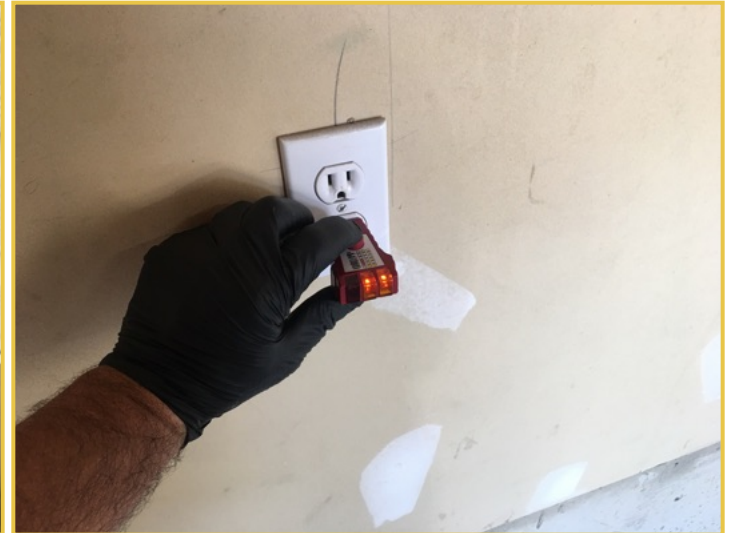
Garage Outlets Not GFCI Protected
