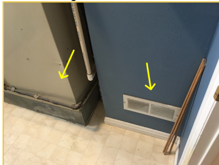
Return Air Within 10 Feet of the Heater
