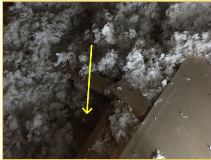
Areas of Missing Insulation
