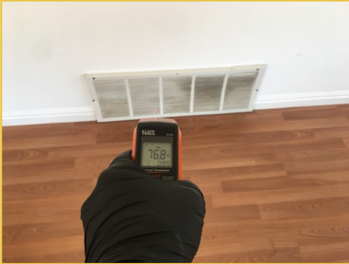
Main Floor Return Air Was at 76 Degrees
