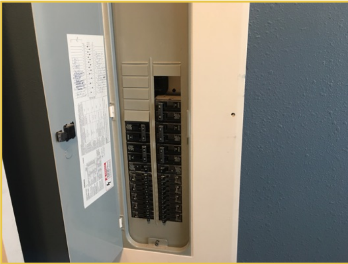
Exterior of Main Electrical Panel
