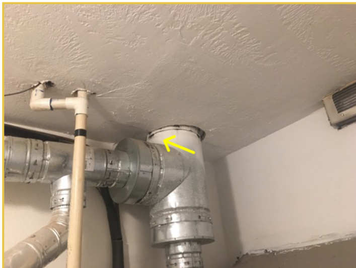
Basement Hot Heater Exhaust Piping In Contact With Combustible Material
