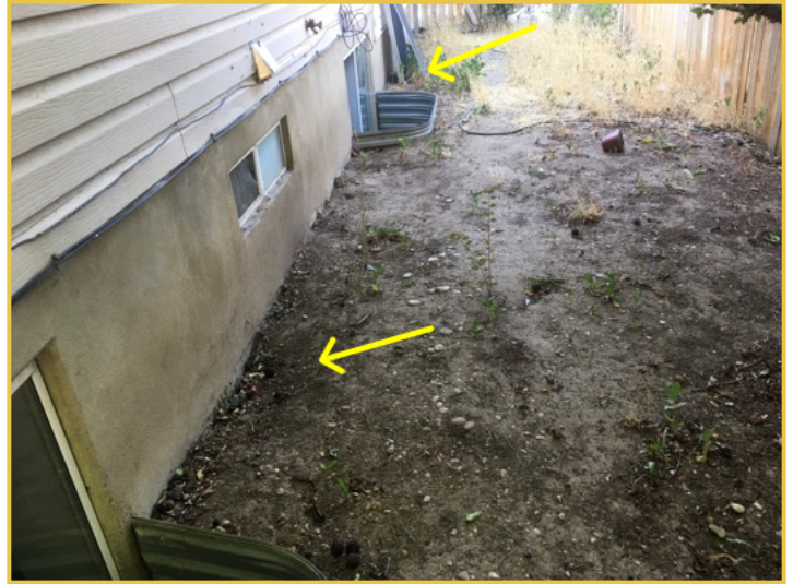
Improperly Sloped Grading
