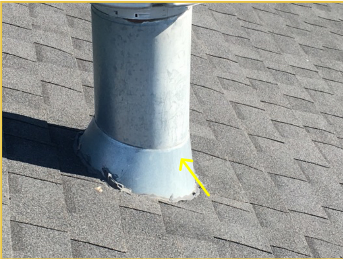
Gap in the Vent
