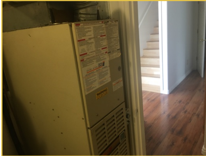
No Green Sticker on the Basement Heater
