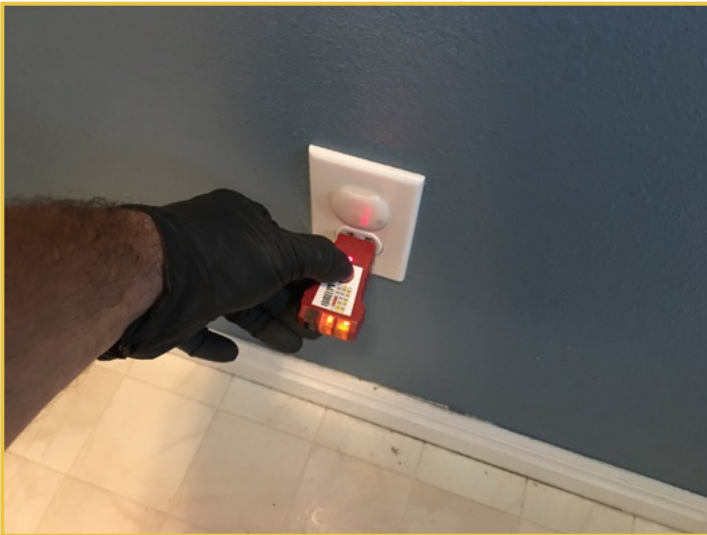
Laundry Outlets Not GFCI Protected
