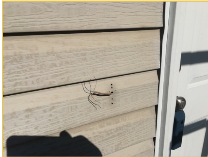
Missing Doorbell Components
