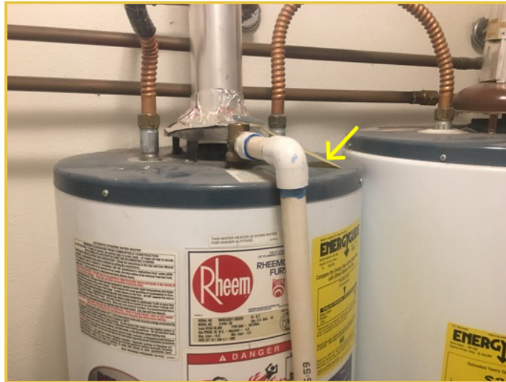
TPR Valve Pipe Not High Heat Tolerant
