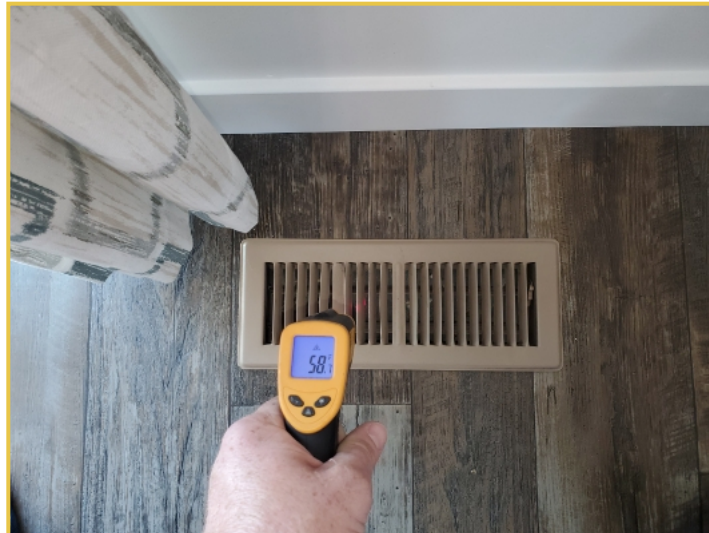
Air Conditioning Ran at 58 Degrees
