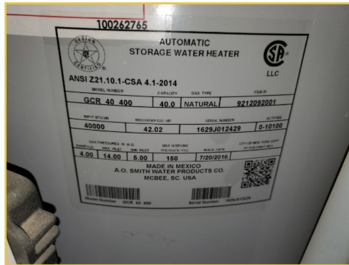
Water Heater Dated July 2016
