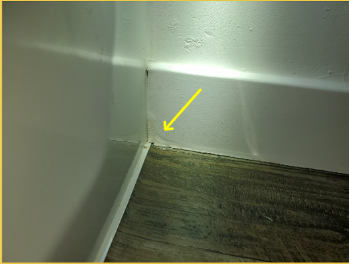
Evidence of Past Leaking at the 2nd Floor Full Bathroom Baseboards That Was Dry
