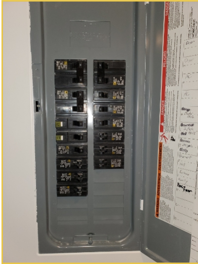
Exterior of Main Electrical Panel
