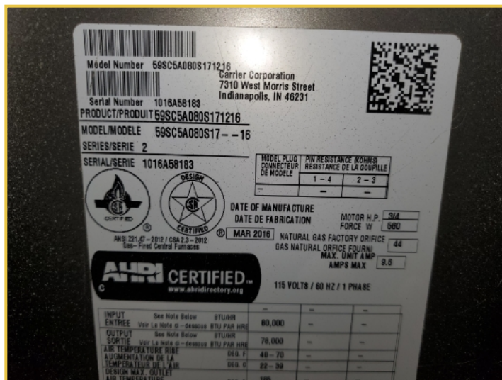
Furnace Dated March 2016
