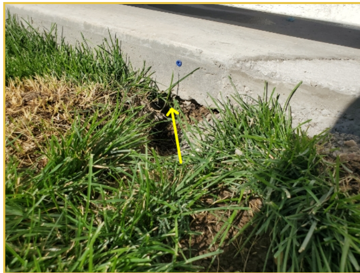
Void Under The Rear Concrete
