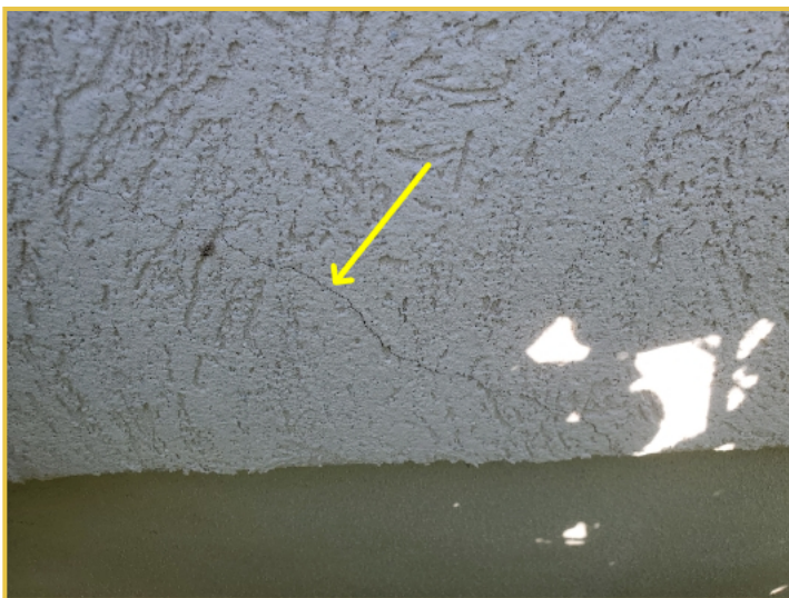
Cracked Stucco Siding
