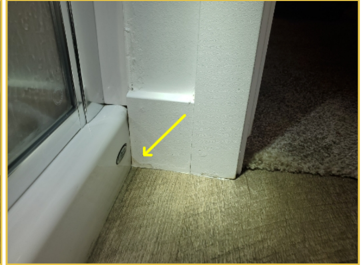
Evidence of Past Leaking at the Basement Bathroom Baseboards That Was Dry
