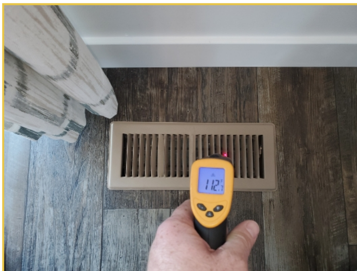
Heater Ran at 112 Degrees
