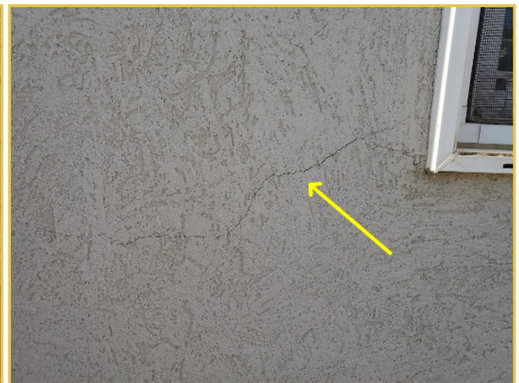
Cracked Stucco Siding at the Window
