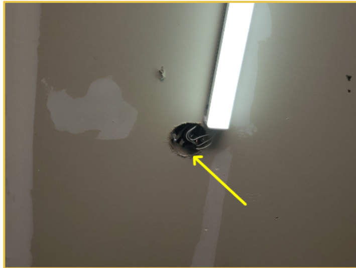
Garage Junction Boxes Without Covers
